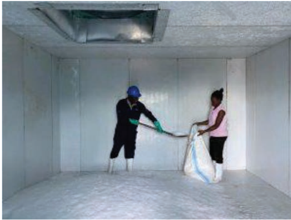
FIGURE 5.3: Ice Manufacturing Unit Powered by Engie-Equatorial's Solar Mini Grid in the Lolwe Islands, Uganda
